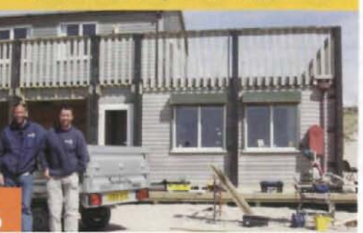
Below: Martin Ward and Greg Spray outside the operations room being built at Perranporth
