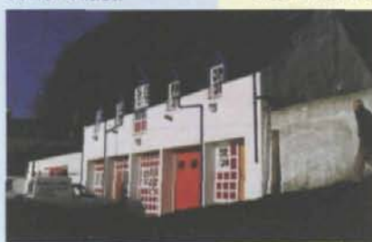
The 1993-built Tobermory boathouse, currently plagued with problems from a nearby sewer outlet.
