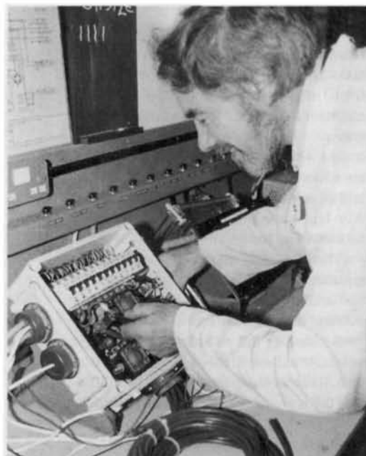
The isolating box, as well as the control panel and the batteries, are made watertight and tested before being fitted into the console by the electricians. Photo Bob Kennovin.
