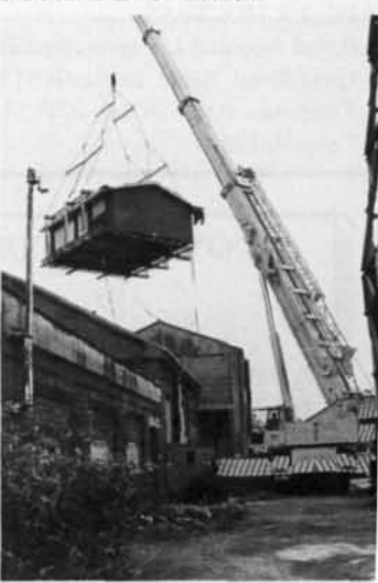
The Barry Dock crew building takes a short cut to its new location.
