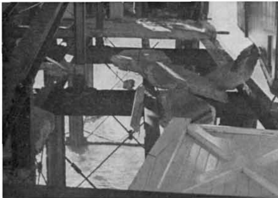
Margate: (Left) With the floor broken up by waves, inside of lifeboat house stands open to the sea. Slipway can be seen on left. photograph by courtesy of Christopher Fright
