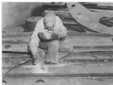
Fig 1: Welding in progress on the workshop floor: (above) the engine bearers are assembled . . .
