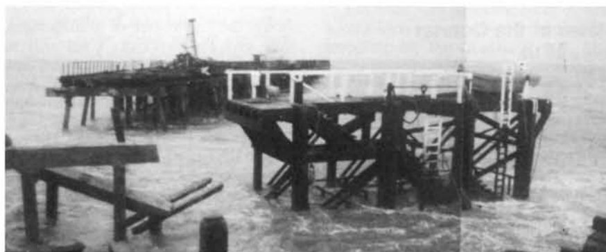
Walton and Frinton: Two photographs taken by Motor Mechanic William Jenkins, put side by side, show the damage inflicted on Walton pier by the storms on New Year's Eve. The landing stage for the station's boarding boat was completely isolated.
