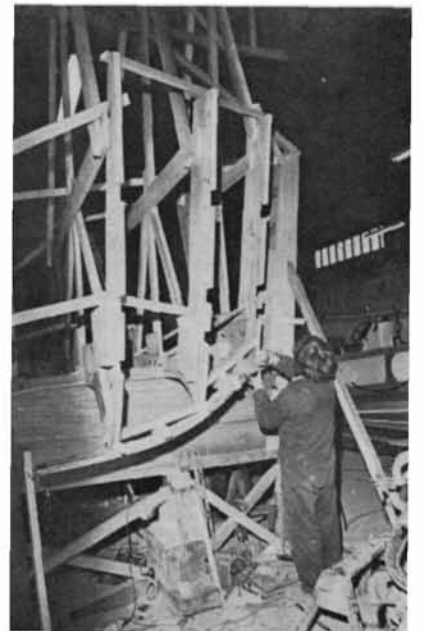
The curved after end of the tunnel cant is built up, in position, of agba laminates scarphed on to solid mahogany for the straight run forward. The building batten can once again be seen at the top of the picture.
