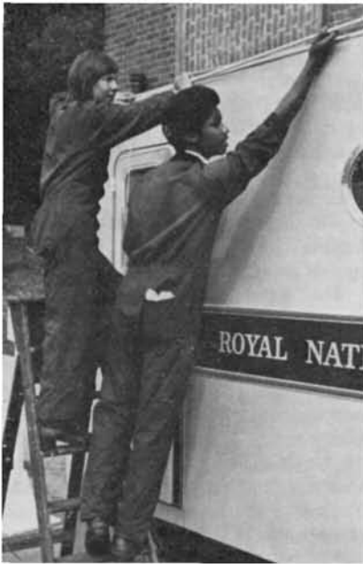
For practical experience, a community service: Two apprentices of the Training Workshops at ICI Fibres, Pontypool, Phil Oakley (left) and Roy Robinson, undertook as their project the wiring-up and commissioning of the electrical/electronics installation of the Mobile Training Unit.
